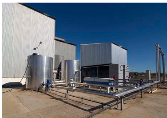
▲ Example of a combined concentrating solar-desalination plant (Almeira, Spain).
