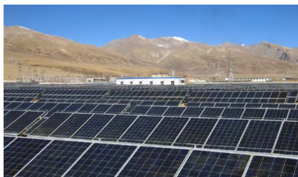
▲ A large-scale (10 MW) array of photovoltaic panels (YangBaJing, Tibet).
