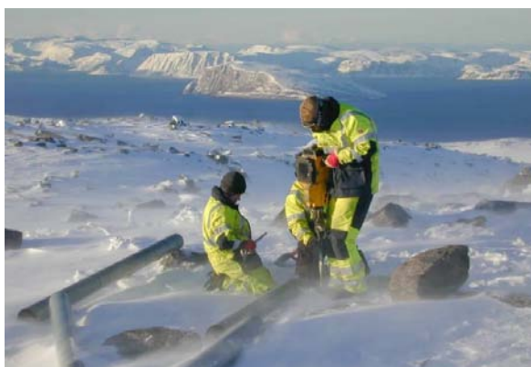
▲ Wind IA Recommended Practices 13 recognises that installing wind turbines in extreme and cold climates requires special equipment, increased focus on personnel safety and expanded planning.
